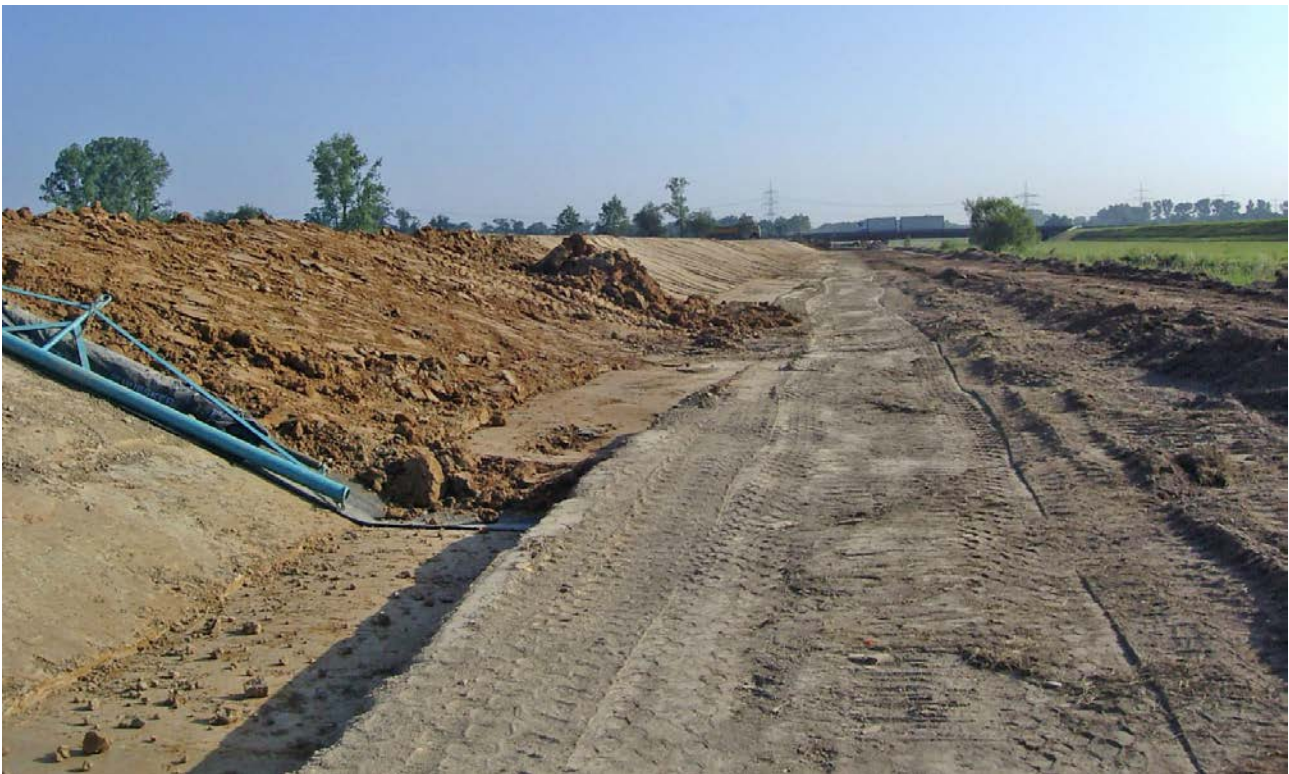
Figure 10: GTD on the Renschflut canal in the installed state
