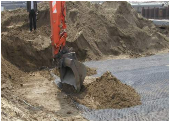
Fig.5 Pretensioning the geogrid by placing a bulg of earth at the end and then pulling it with the excavator shovel
