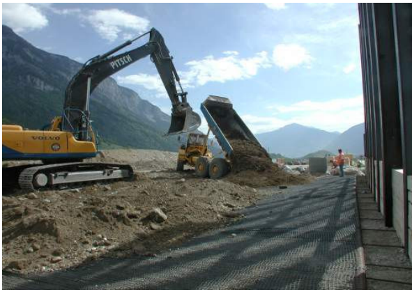
Fig 2. Refilling the first Fortrac® layer, the flexibility of the geogrid is important for a good connection
