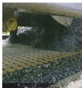
Above right and below: Installation of the asphalt surface course on asphalt reinforcement
