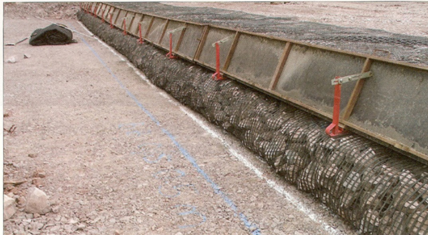
The temporary climbing shutter system used to support the face ensures a tight wrap construction
