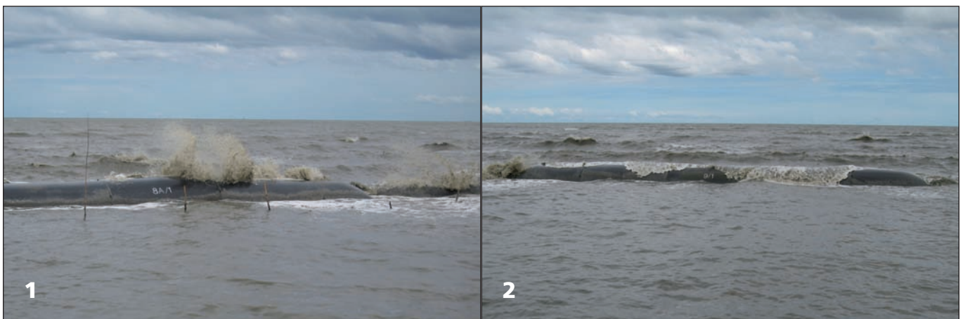
Picture 1/2: SoilTain® Tubes as breakwaters temporarily protruding from the water under wave action during low tide
