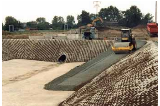
Attenuation pond with Incomat® Crib after apertures have been filled with soil (2)
