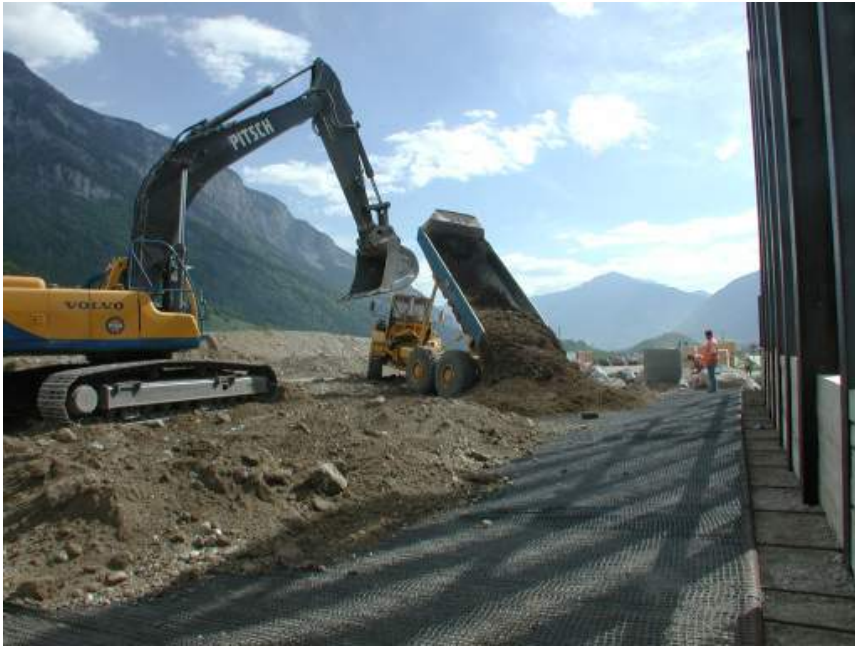
Figure 6. Refilling the first Fortrac® layer, the flexibility of the geogrid is important for a good connection (photo: Schoellkopf)
