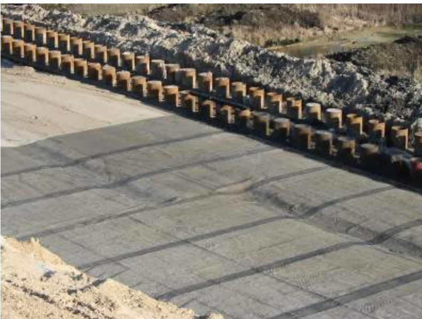
Figure 8. Placed geogrids connected to the two rows of steel tubes (photo: Möbius)
